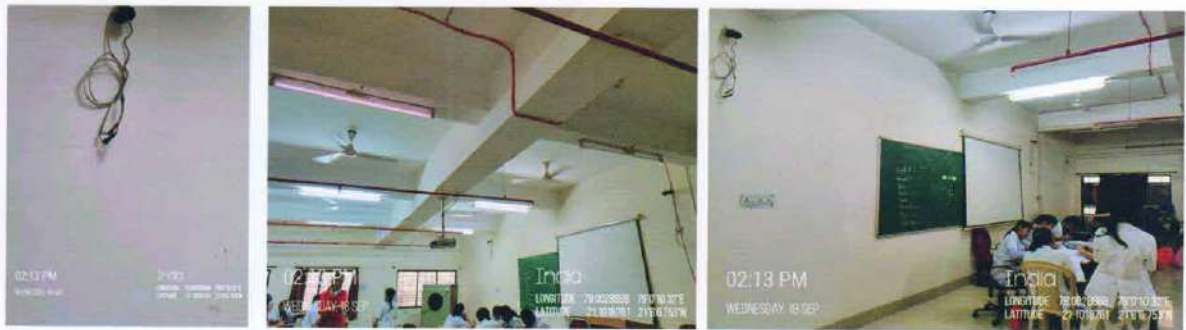
Cameras installed in Lecture Halls
