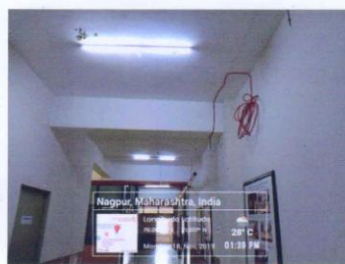
LED Lights in Corridor
