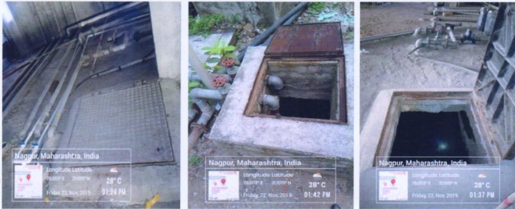
Underground water tanks in campus
