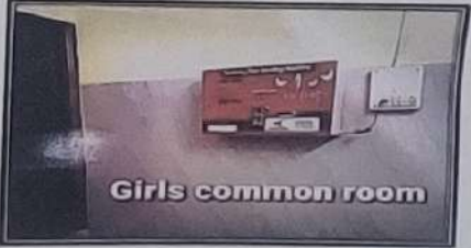
Installed at Girls Common Room
