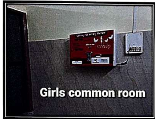
Installed at Girls Common Room
