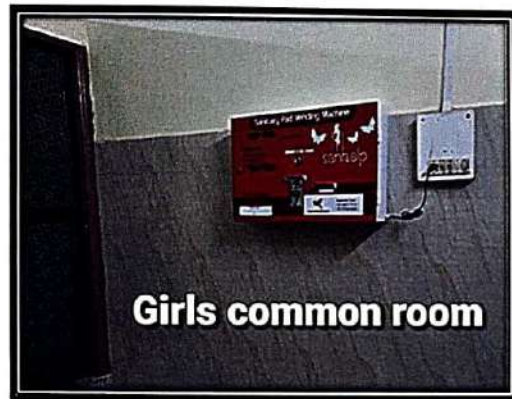
Installed at Girls Common Room
