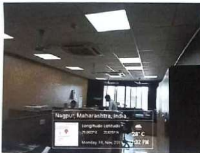
LED Lights in Office
