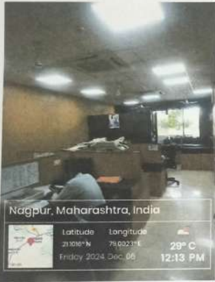
LED Lights in Office
