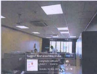
LED Lights in Office
